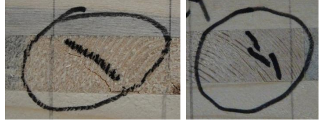
Figure 7: Rolling shear cracks in the trapezoidal fatigue loading test (black marker line in the circle is next to the crack)
