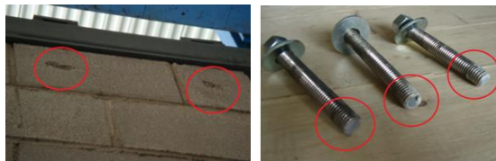
(a) Local crack of masonry block and bolt broken
