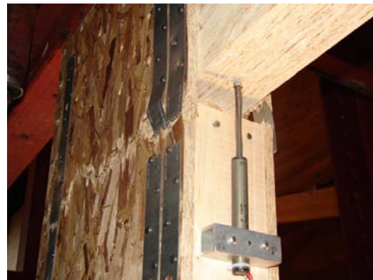
a) Panel shearing and metal strap broken
