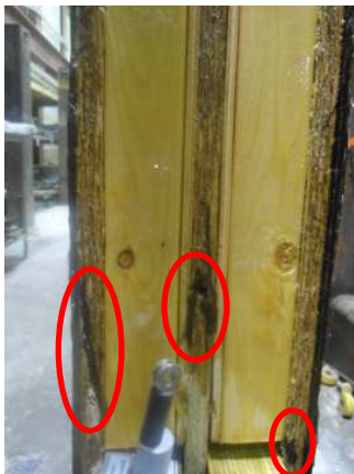
(c) Failure of exterior OSB in FRP-3
